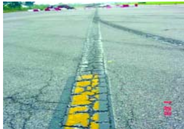
Photograph 8 – Discontinued path marking.
